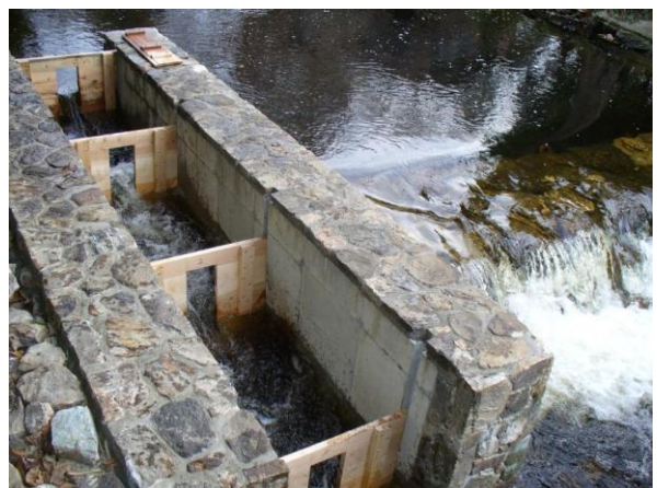
There is a six-inch drop at each of the wooden weirs inside the Fishway. The wooden gate to close the fishway is resting on top of the fishway. One can see the stone façade added to cover the concrete walls.
