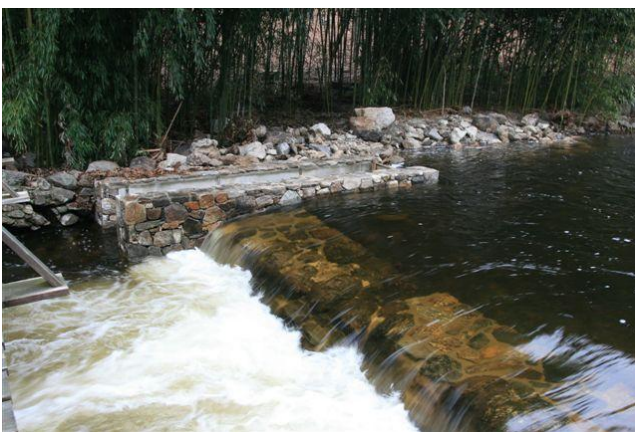
The completed Grossman Fishway as seen from the far bank. This photo was taken in high water and the dam looks passable but at typical flows, this dam blocks fish runs. The right bank fishway allows fish to pass while blending in to the surrounding landscape.
