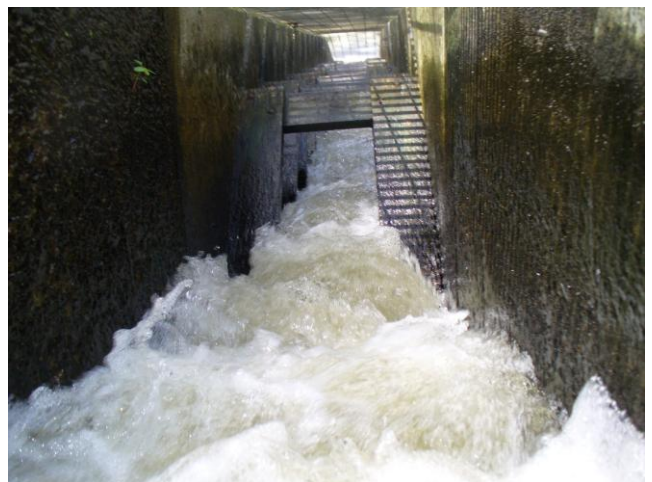
A look at the inside of the fishway with its wooden baffles.
