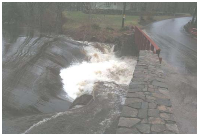
The Rathbun Dam (upstream of the Moulson Pond fishway on the Eightmile River) in Lyme. There's normally about a 20 foot gap between the bridge and the water surface below.
