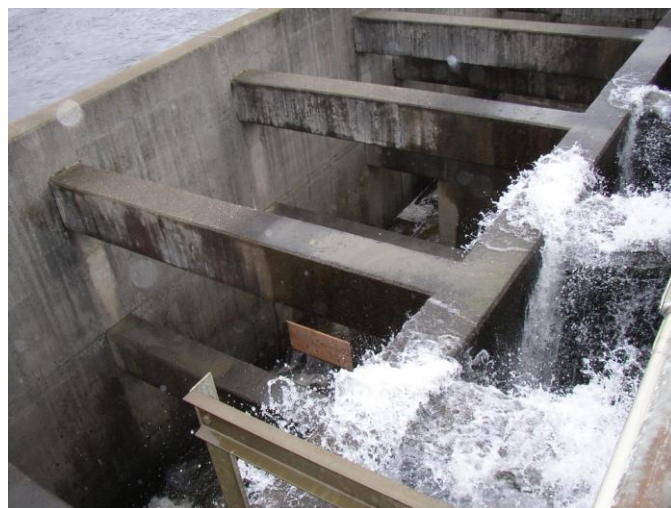
The same area of the Vernon Dam as shown to the left, but with a missing weirboard replaced with new wood. The notches above and below this notch do not have boards because the blocked notches are staggered from one side of the fishway to the other. Only the notches on the far side are visible in these photos; the other side is hidden by the inner wall that runs parallel to the outside wall.
