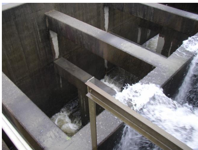
The lower section of the Vernon fishway with minimal flow showing missing boards across weir notches. In the photo to the right, you can see new wooden boards inserted into steel channels. These boards block off one notch of two on each weir to create favorable hydraulics. With these boards missing, water spilled through both notches, creating turbulent flow not favored by American shad (Photos by Jay McMenemy, VTFG).
