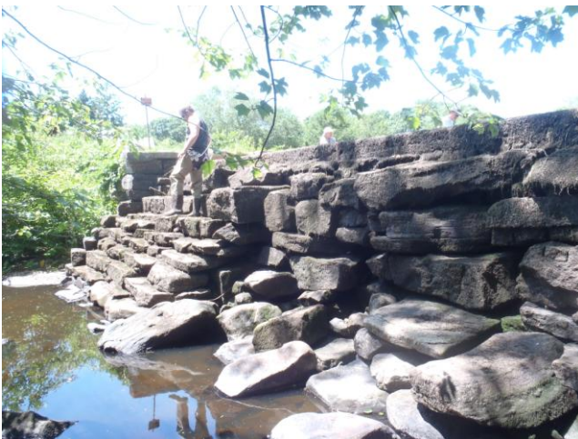
The Rutan Dam is not that old but is in very bad shape. Removing this dam will reconnect the upper part of the Anguilla Brook watershed with the lower part.
