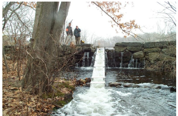
Perhaps the smallest fishway in CT: The Hummers Pond Fishway on Fence Creek in Madison started life as one of our earliest ones made out of wood but replaced with aluminum. It gets a call out this week because it appears that a wave of alewives have gone up it this past week!
